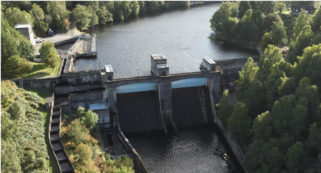
Clunie Dam in Scotland, digitally inspected with the help of STRUCINSPECT. © STRUCINSPECT
